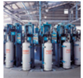
LPG Filling System
