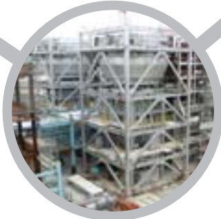
Rotating-type surface melting furnace
