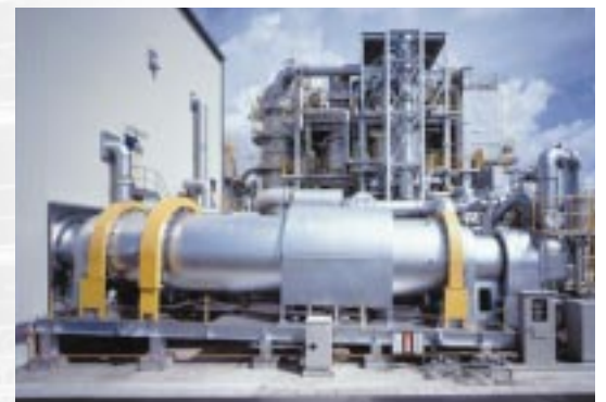
Gasification and melting furnace
