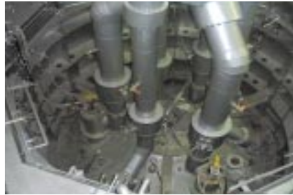
Rotating-type surface melting furnace
