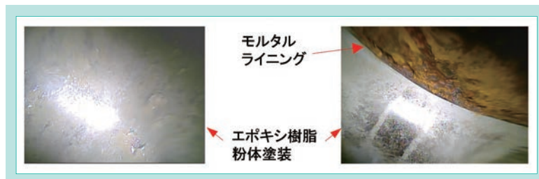
図 18 エポキシ樹脂粉体塗装の状況 Fig. 18 Fusion Bonded Epoxy Resin Powder Coating Under Corrosive Environment
